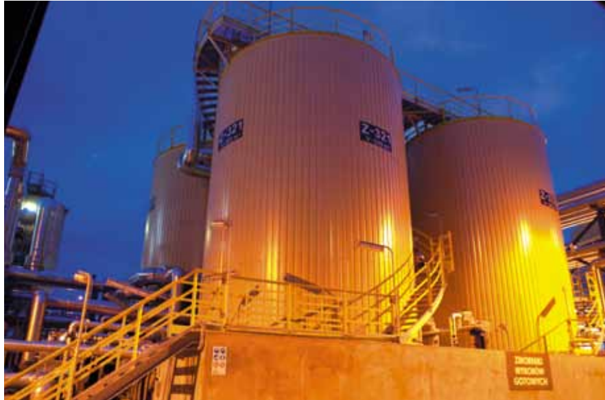
Figure 9.3. Modified-bitumen tanks, Płock site (photo by ORLEN Asphalt sp. z o.o.)
