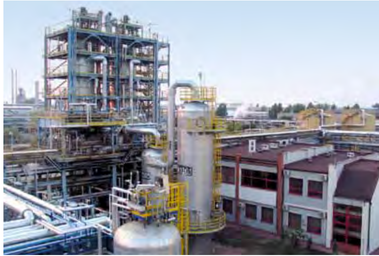
Figure 1.2. Continuous oxidation system – Biturox® reactors (photo by ORLEN Asphalt)
